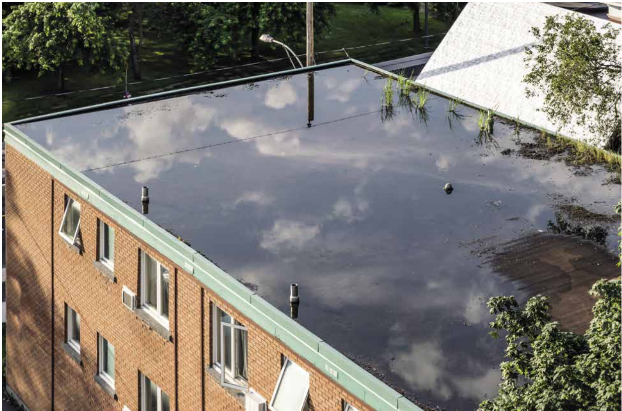
Figure 1: Ponding on a typical flat roof
