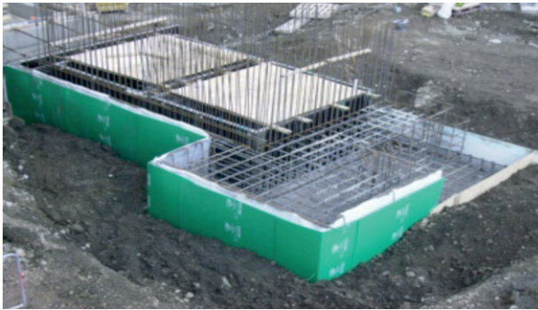
BRADFORD PARADE CITY CENTRE Retail shopping and office developments waterproofed due to high watertable.
