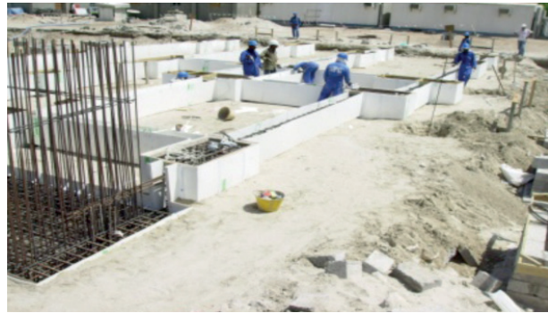
ABU DHABI HOUSING PROJECT Pile caps and ground beams installation Proofed to resist sulphate attack.
