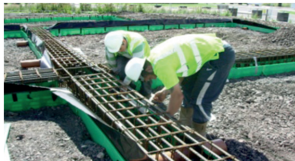
ROB ROYSTON, SCOTLAND 5 STOREY OFFICE DEVELOPMENT Attaching gas membrane starter strip to ground beam.
