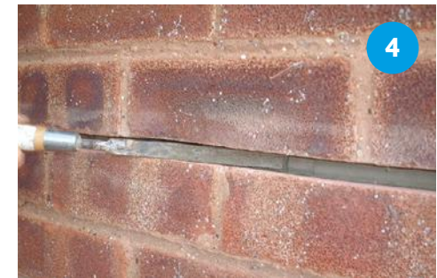
Make good the wall chase to disguise the slot. Repair cracks between the helically reinforced masonry with Crack Sealer Plus.
