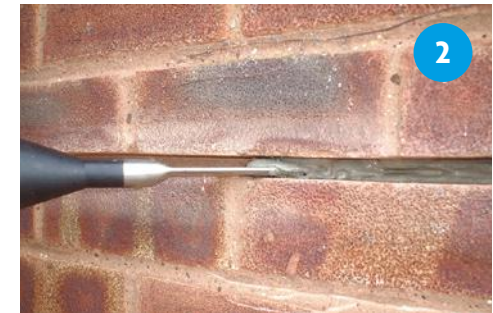
Clear loose debris from slots and flush thoroughly with water and insert bead of WHO 60 grout.
