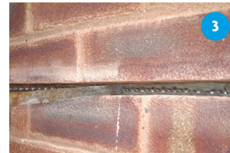
Push helical crack stitching bar into grout, to approximately two thirds of the slot depth. Trowel displaced grout to firmly encapsulate the bar.
