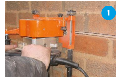
Chase horizontal slots at 300mm intervals that extend 500mm on each side of the crack.
