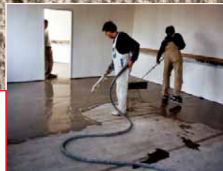
MAGNA STEYR GROUP PLANT - Graz - Vienna Substrate preparation with: NIVORAPID, ULTRAPLAN, PRIMER G. Installation of linoleum with AQUACOL T
