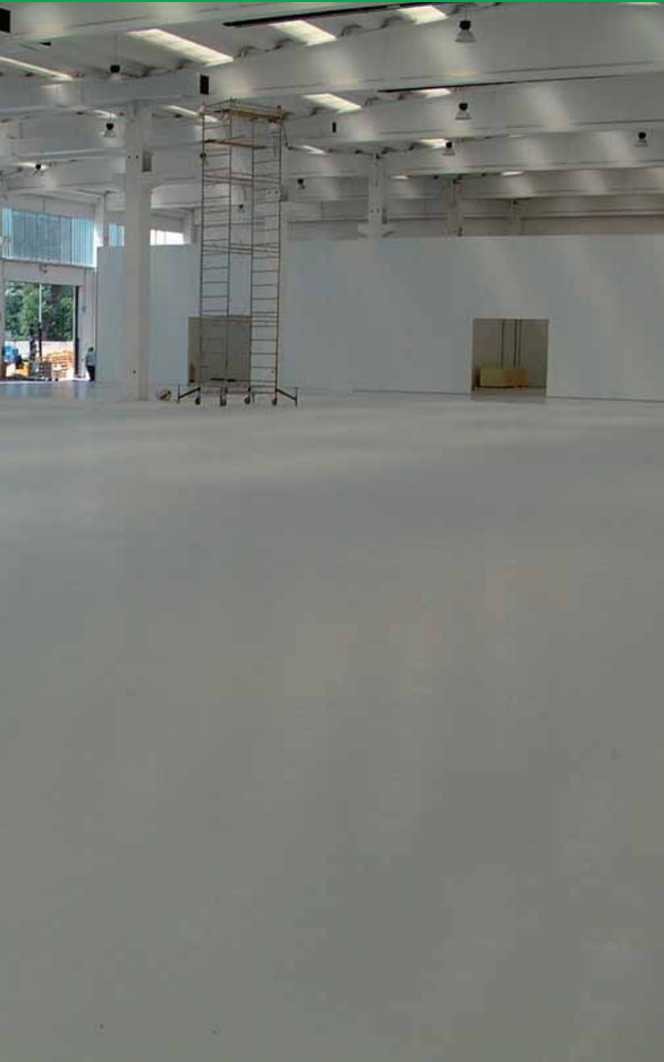
MANCINELLI LOFT BUILDING - Tribiano (MI) - Italy Covering new concrete flooring with: MAPEFLOOR SYSTEM 33 (PRIMER SN, MAPEFLOOR I 300 SL, MAPECOLOR PASTE, 0.25 QUARTZ, 0.5 QUARTZ, MAPEFLOOR FINISH 51)
