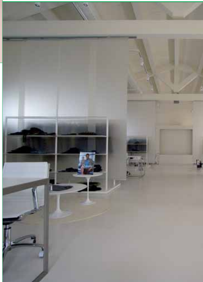
Ingram show-room - Arezzo - Italy Repairing of flooring with: ULTRATOP SYSTEM "natural effect" ( PRIMER SN , ULTRATOP , MAPEFLOOR FINISH 52 W )
