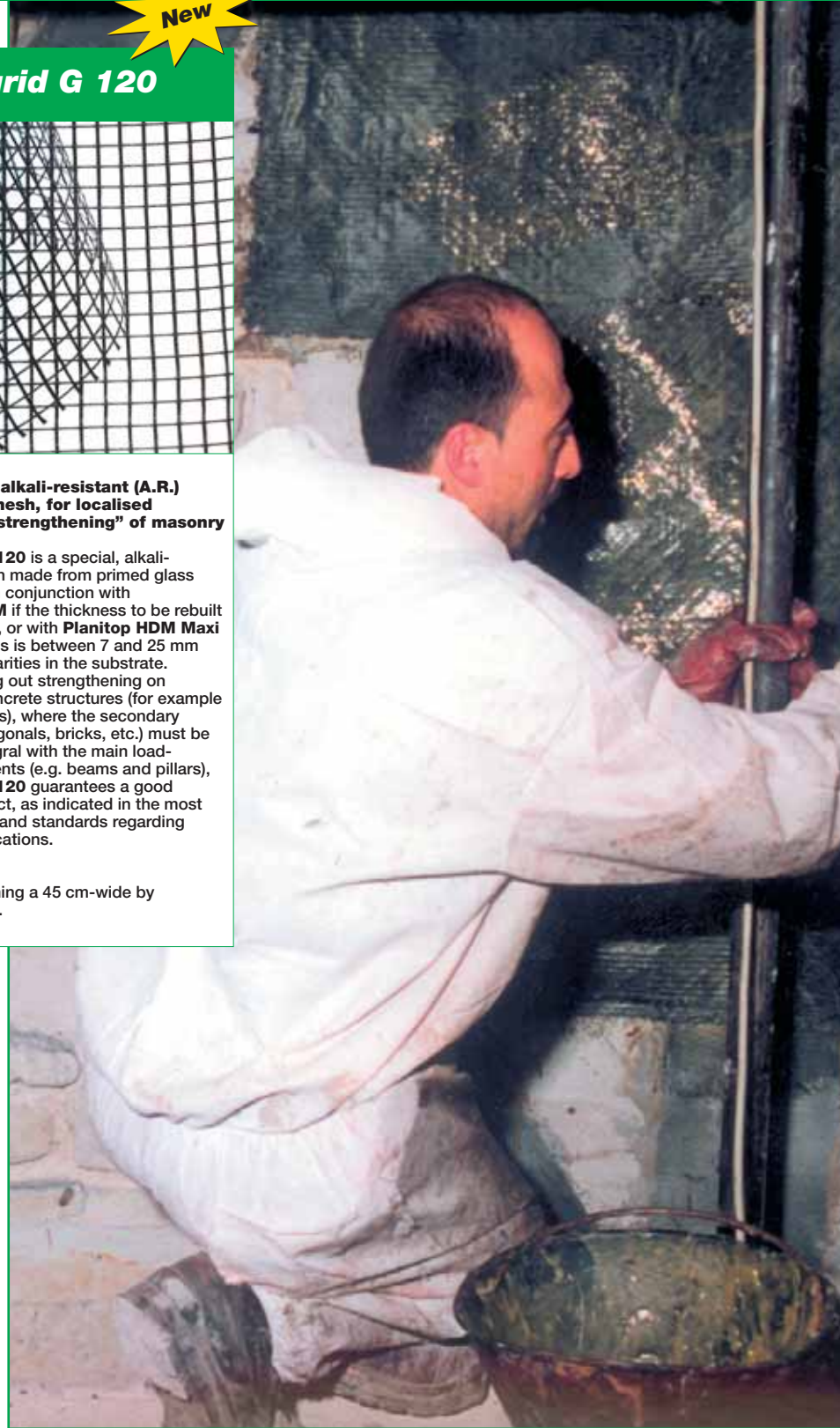
Church of St. Lucia Bell-tower - Serra S. Quirino - Ancona - Italy Consolidation and of the concrete structure using: MAPEWRAP PRIMER 1, MAPEWRAP 11, MAPEWRAP 31, MAPEWRAP C UNI-AX, MAPEWRAP C QUADRI-AX, ADESILEX PG1, EPOJET, MAPE-ANTIQUÉ MC and ANTIPLUVIOL S
