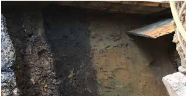
HYDROCARBON LAYER FOUND AT RESIDENTIAL PROPERTY
