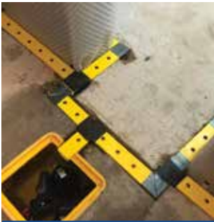
DELTA SUMP PUMP / CHANNEL CONFIGURATION
